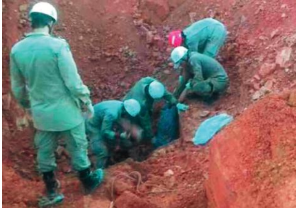
Figure 4 Photo of the trench slip, which victimized the geologist (24 horas news, 2017).
